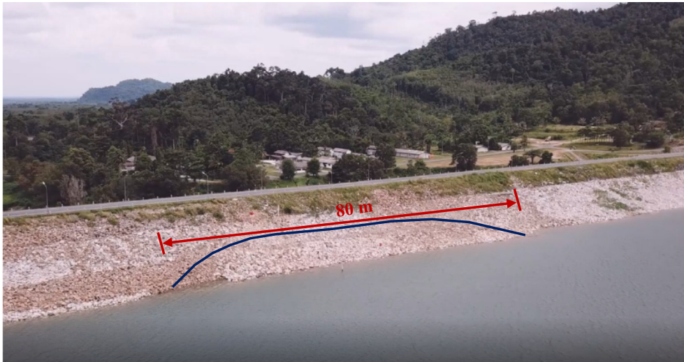
Fig. 2. Observation of a crack at the upstream slope of Khlong Pa Bon Dam (Royal Irrigation Department 2016).
